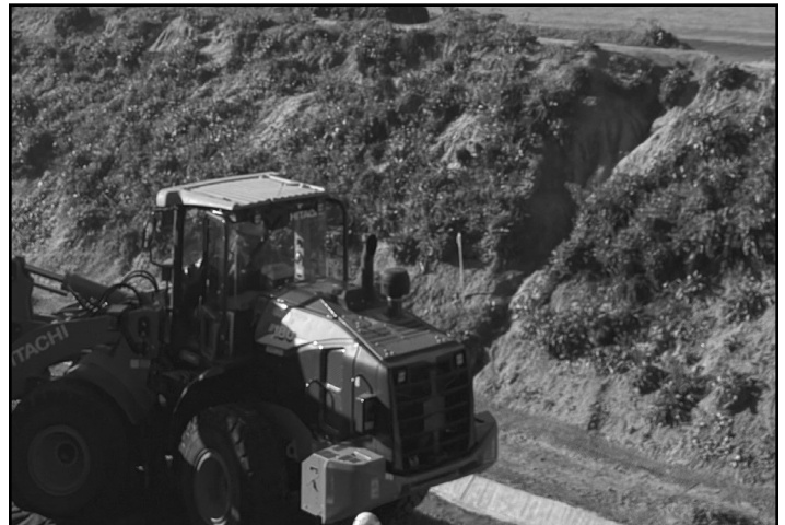
Bluffs work; More concrete poured into forms are set together parallel to protect the track.. Photo: Julie Maxey-Allison
