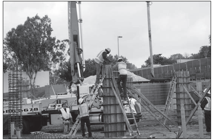
Pumping concrete into column forms to support upper deck. Photo Don Mosier.
