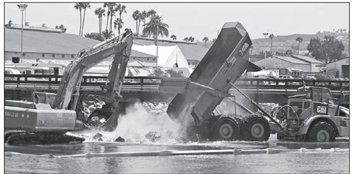
Another noisy activity next to the Fairgrounds - shoring up the timber train trestle with rip rap. Photo Bill Morris
